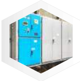
INDUCTION MELTING FURNACE
