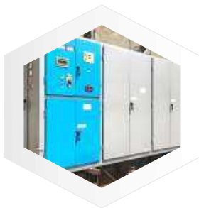
INDUCTION MELTING FURNACE
