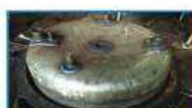
Gas Carburising Furnace
