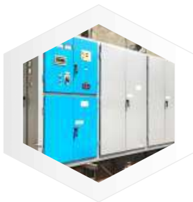
INDUCTION MELTING FURNACE
