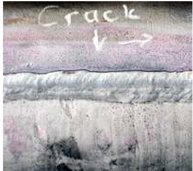
Crack During Welding
